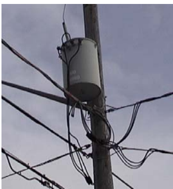
Foto.A Monophase transformer MV/LV
